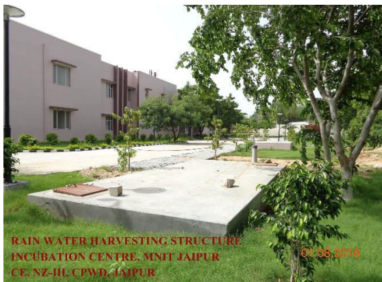
Rain water harvesting system at MNIT Jaipur
